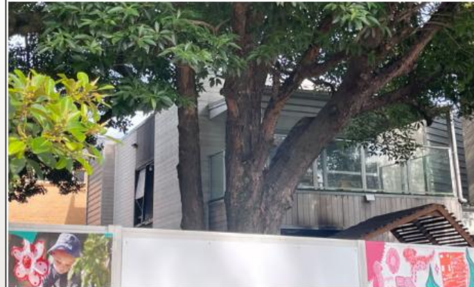
📷 Damage at the scene of a fire at a childcare centre in Maroubra in Sydney Photograph: Daisy Dumas/The Guardian
